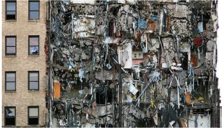
Figure 9. Partially demolished Children’s Hospital Pittsburgh PA and its variety of modern construction materials
